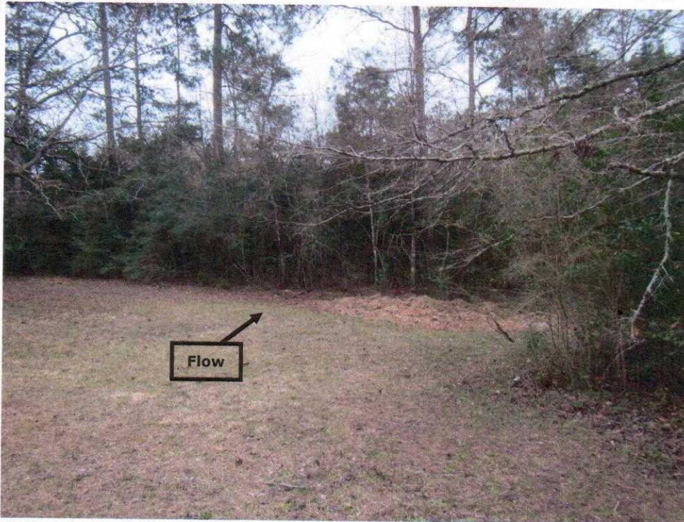
Photo 16: View of the emergency spillway entrance, from the left/upstream corner of the service spillway chute, facing downstream (southeast). Note that the channel is lined with thick tree growth that would impede flow.
