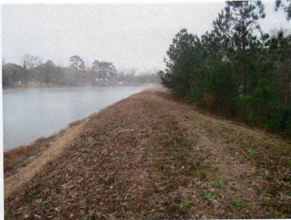
Photo 1: View of the dam crest, from the right side of the dam, facing left (east). Note the fair grass cover and animal trail/foot path.
