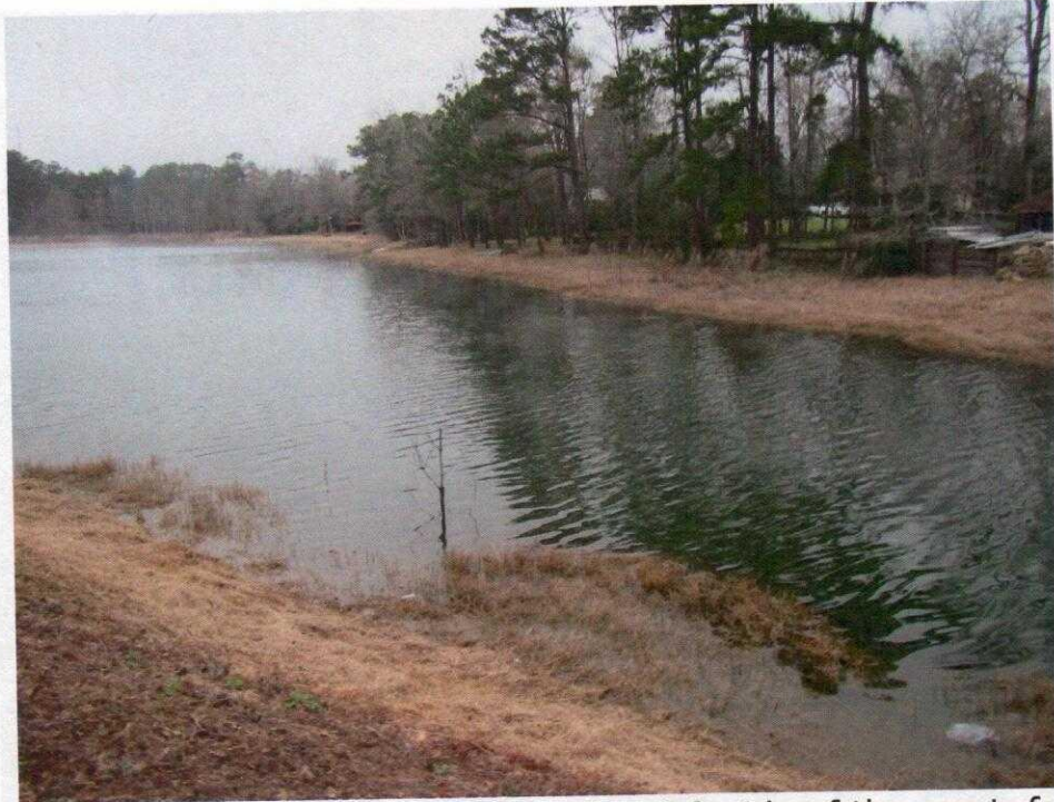
Photo 5: View of the reservoir from the left side of the crest, facing northwest. Note the trees growing near the upstream toe (only the top of the tree is above the water line).
