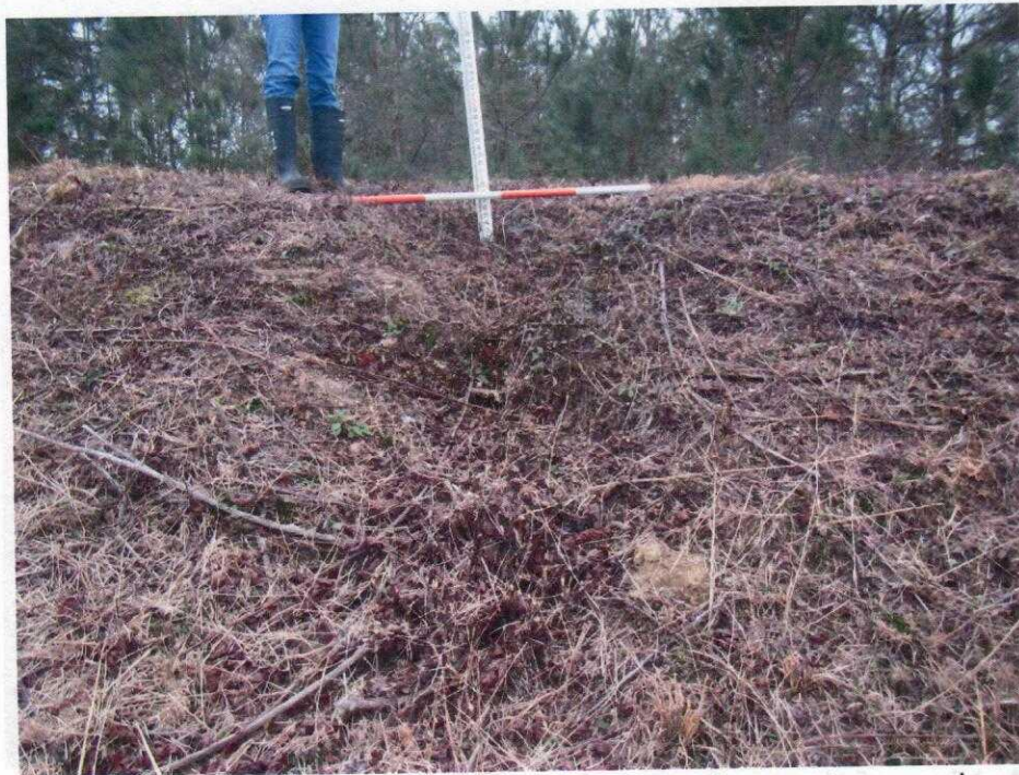
Photo 6: An example of the erosion gullies in the upstream slope at the crest shoulder. This example was 4-ft. wide and 0.7-ft. deep, on the left side of the dam, facing downstream (south).
