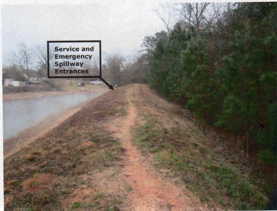
Photo 2: View of the dam crest, from the left/middle side of the dam, facing left (east). Note the fair grass cover and more defined animal trail/foot path compared to the path in photo 1.
