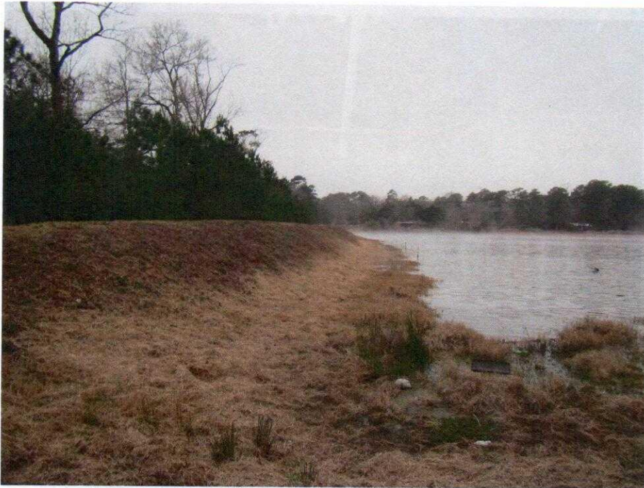
Photo 4: View of the upstream slope, from the left end of the dam, facing right (west). Also note that the upstream slope had been cleared of brush and trees and had a fair grass cover.
