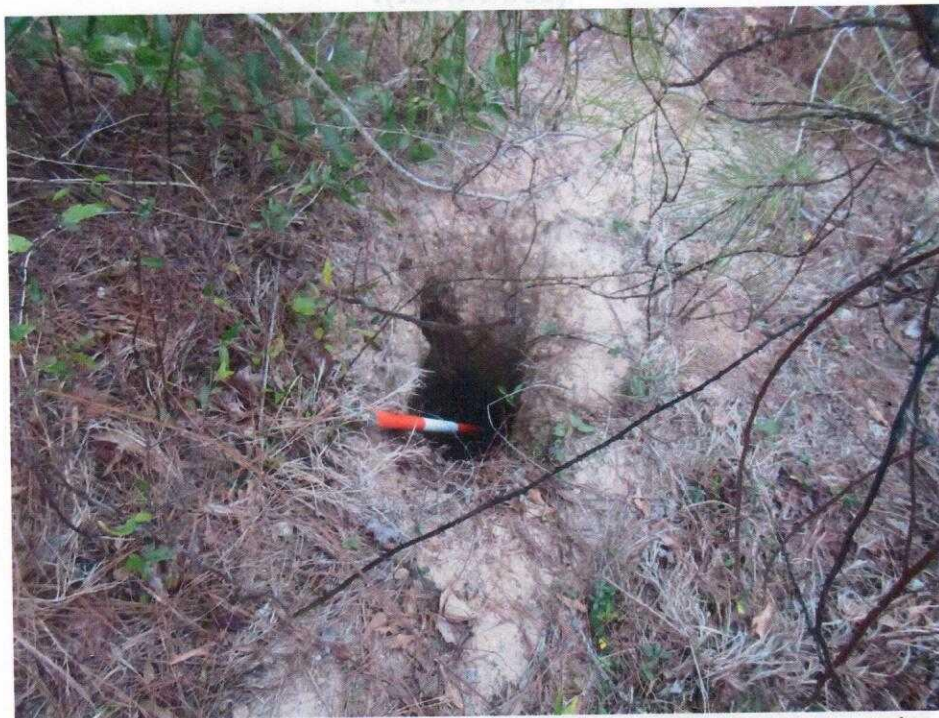
Photo 14: An example of the holes found in the downstream slope. This example measured to be 3-ft. wide and 4-ft. deep. This photo was taken on the right/middle side of the dam, facing upstream (north).
