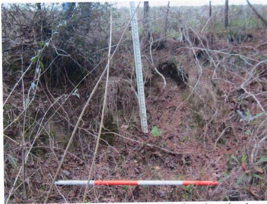
Photo 13: An example of the erosion gullies found on the downstream slope. This example measured approximately 4-ft. wide and 3-ft. deep. This example was found near the middle of the dam, facing upstream (north).
