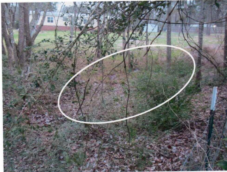
Photo 9: View of the seepage area (circled) that triggered the complaint inspection, on the right side of the downstream toe, facing downstream (southwest). Note that the area was fenced off, so the origin of the seepage was not closely inspected.
