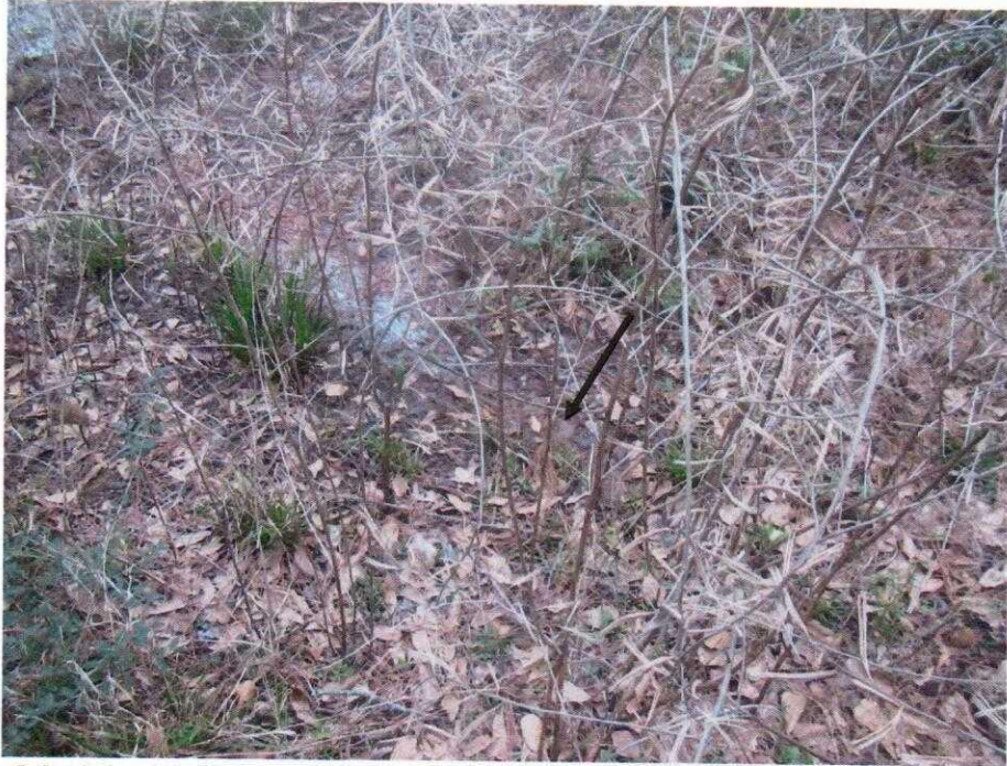
Photo 11: View of the seepage (arrow) emerging from the downstream slope, approximately 3-ft. up the downstream slope from the toe. This photo was taken on the right side of the downstream slope, facing downstream (southwest).
