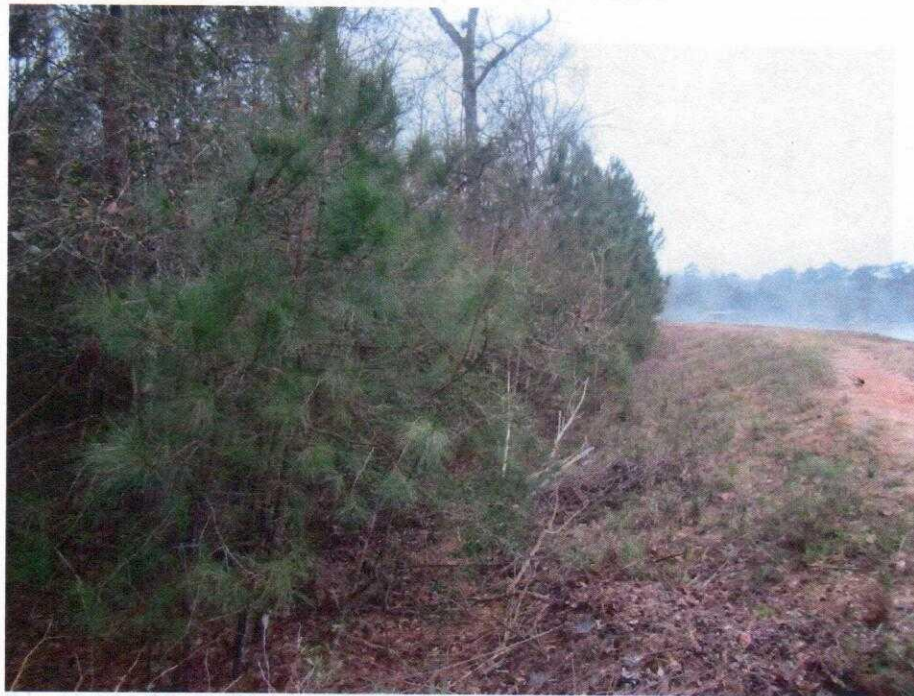
Photo 8: View of the downstream slope, from the left end of the dam, facing right (west). Note the thick tree and brush growth along the lower two-thirds of the slope and downstream area.
