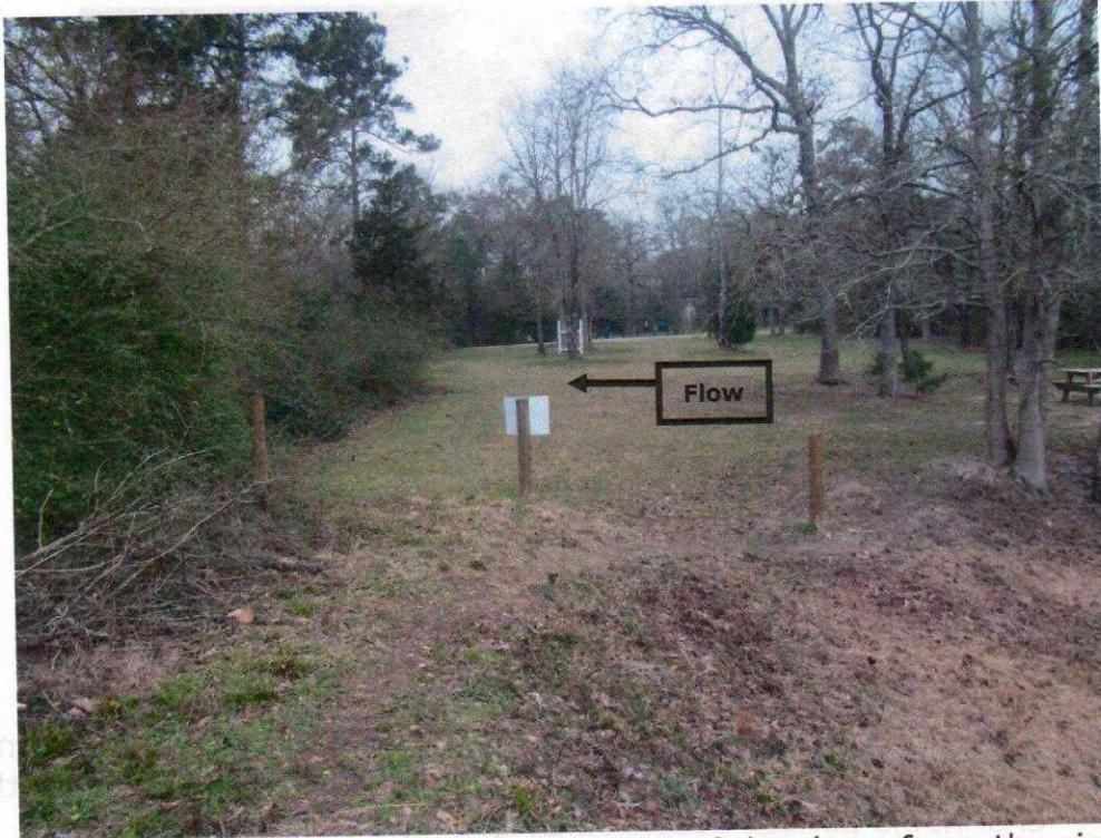
Photo 17: View of the low area to the right of the dam, from the right end of the crest, facing right (west). Note the trees in the immediate channel.
